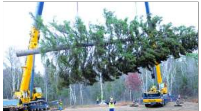
A crane was used to hold the tree upright as it was cut. A second crane lifted the bottom of the tree for loading onto a specially-equipped truck.
